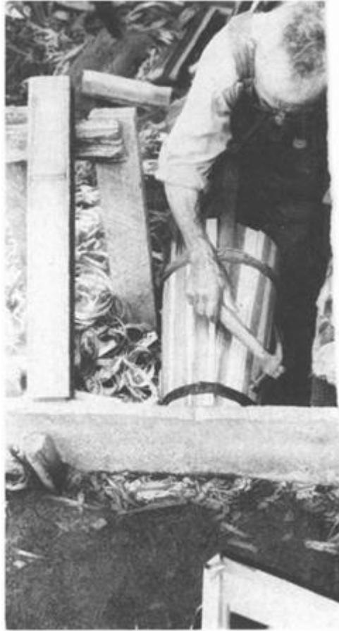
ILLUSTRATION 18 Step 5: Use a hammer to fit in the last stave. If it won't fit, adjust the other staves with the jointer. A tight fit is absolutely necessary.
